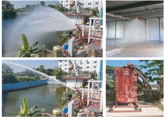
Fixed Fire Fighting Installations at IMA Fire Fighting training school: Foam System (Spray and Jet Mode), Hyper Mist system & Dry Powder system.
